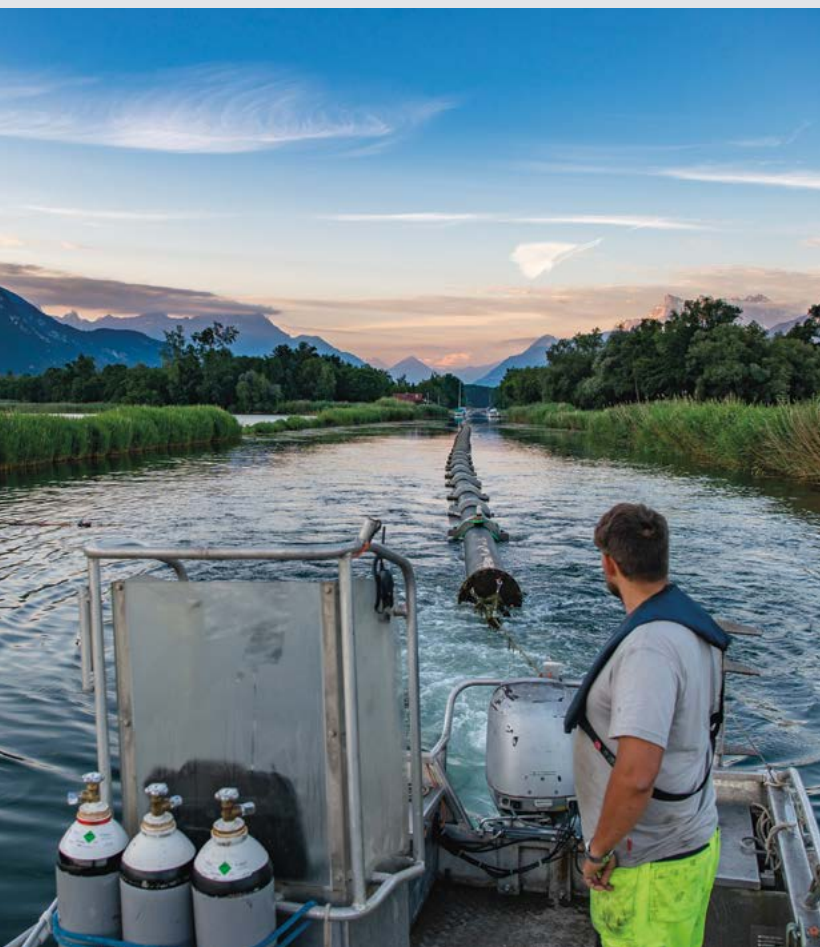
▲ Water pipe for International Olympic Committee HQ in Vidy (Switzerland)
